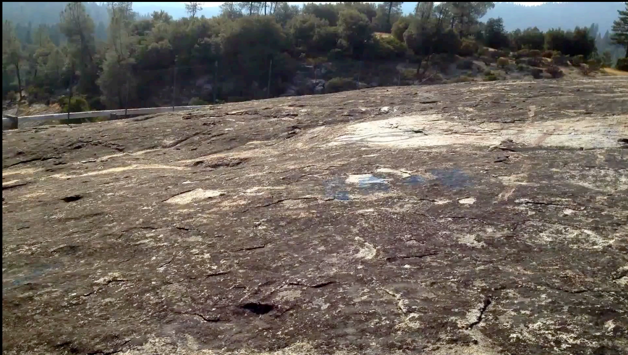
Twain Harte Dam Rock Exfoliating (Colins+18)
